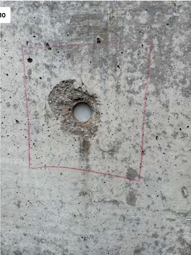
View of Spalling.
