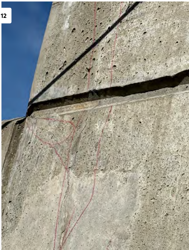
View of Concrete Crack.
