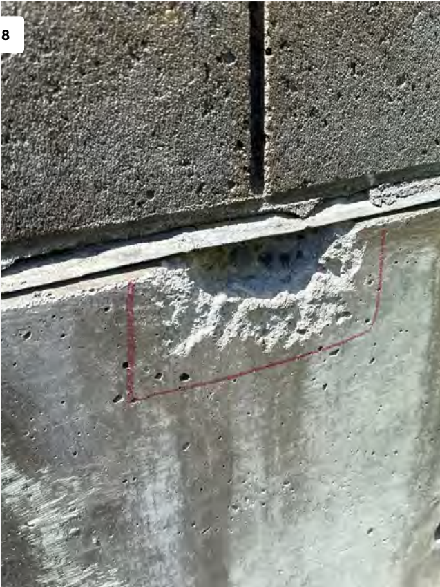
View of Concrete Damage.
