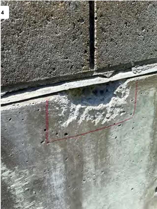
View of Concrete Patch Requiring Further Exposure
