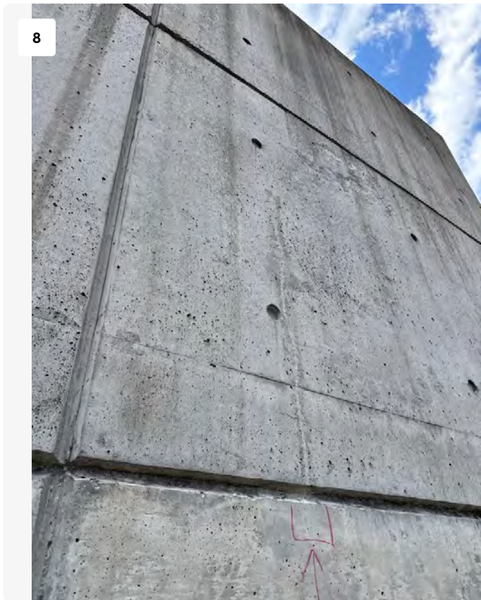
View of Portion of Crack Repaired. Re-Rigging is Required to Repair in its' Entirety.
