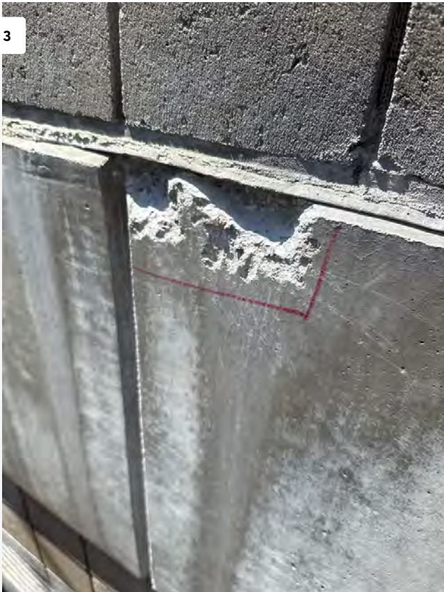
View of Concrete Patch Requiring Further Exposure
