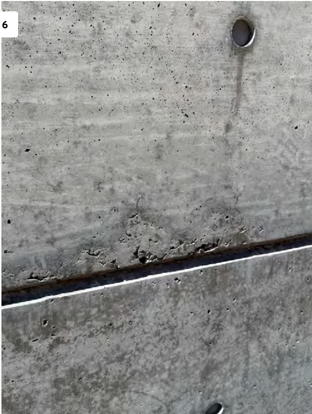
View of Honey Combed Concrete
