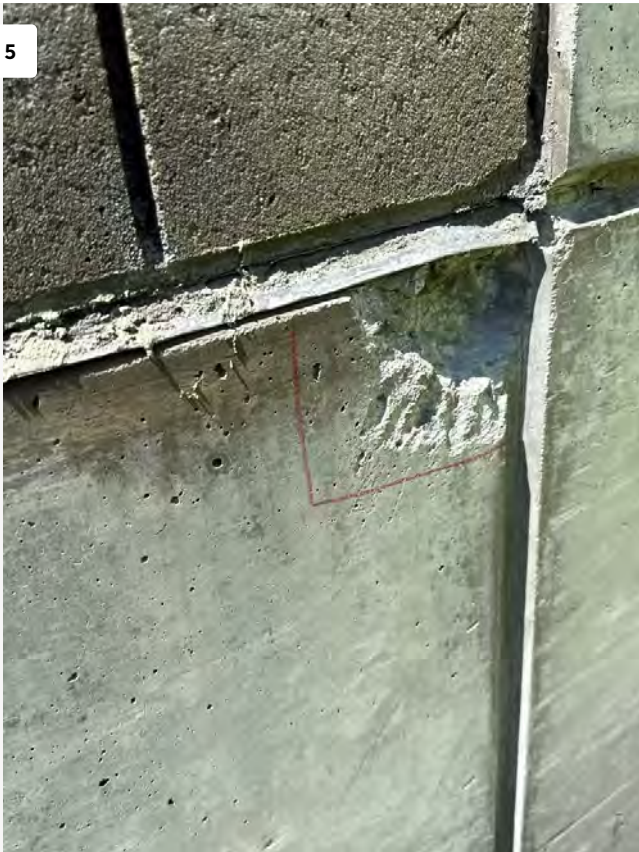
View of Concrete Patch Requiring Further Exposure
