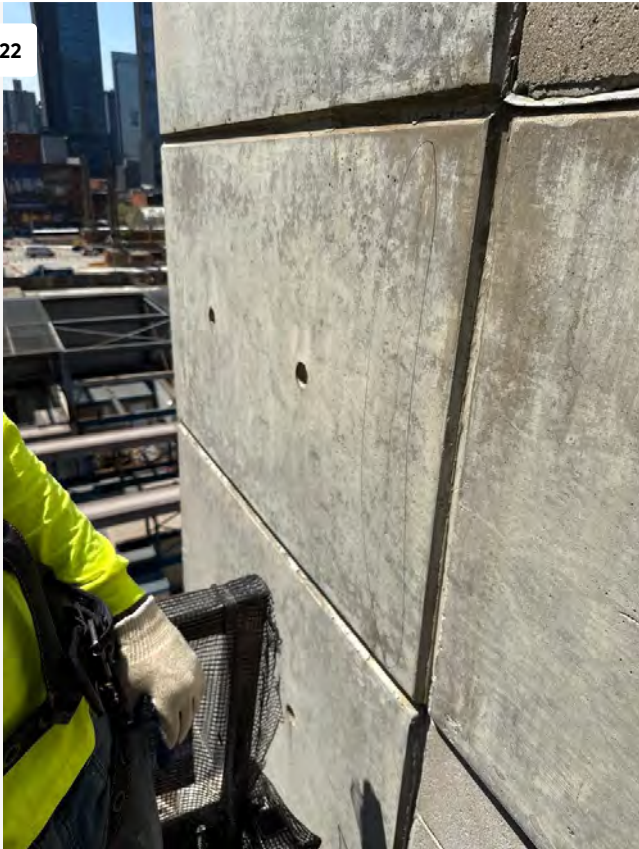
Crack at East Elevation
