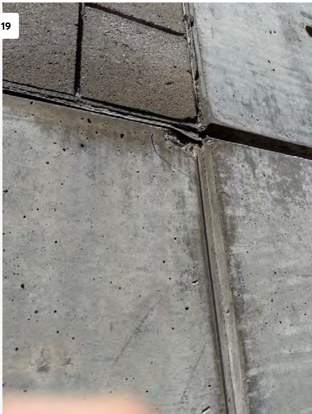
Spalling at East Elevation
