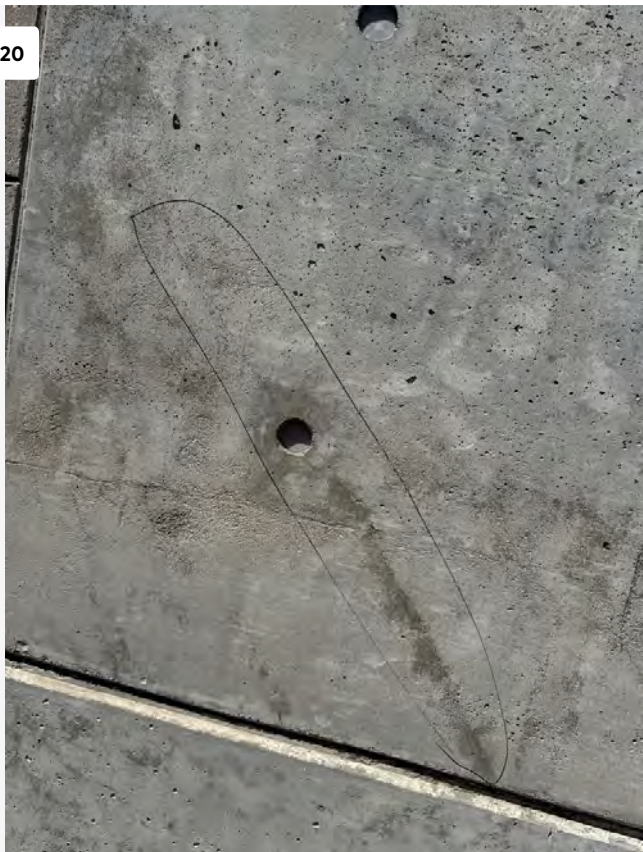
Crack at East Elevation
