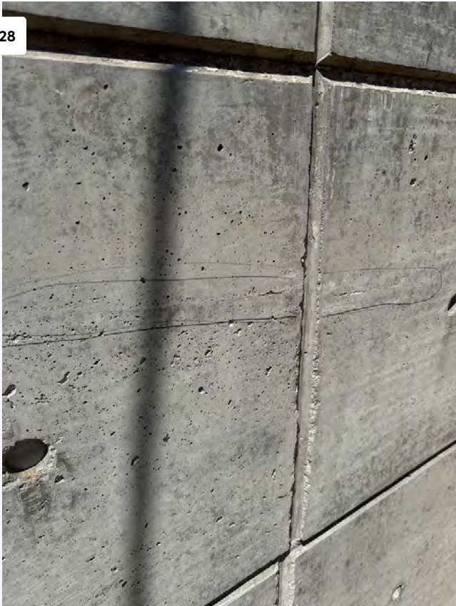
Crack at East Elevation
