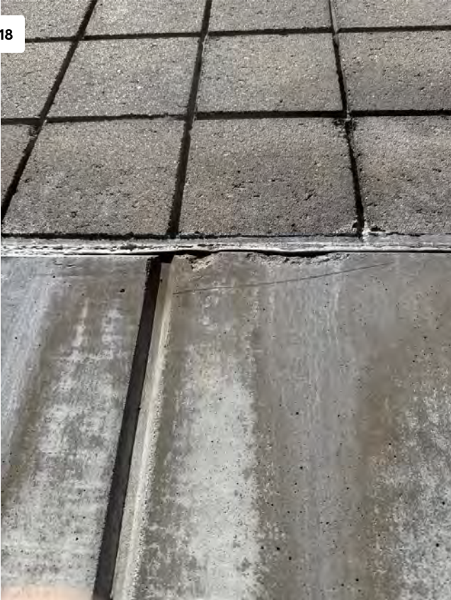
Spalling at East Elevation
