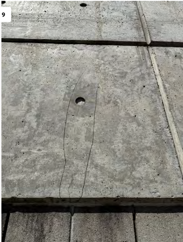
Crack at East Elevation
