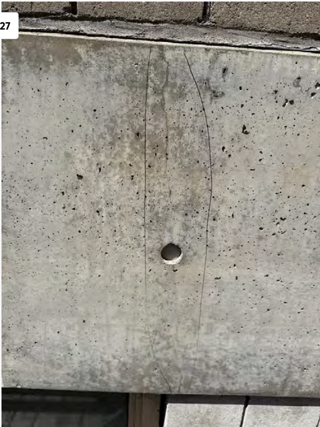
Crack at East Elevation
