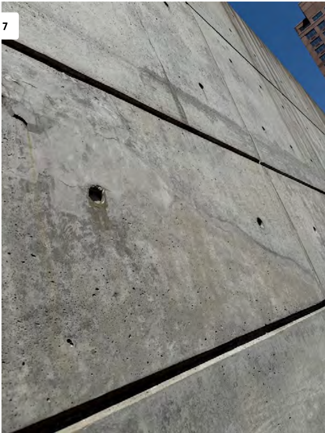
Discoloration at East Elevation
