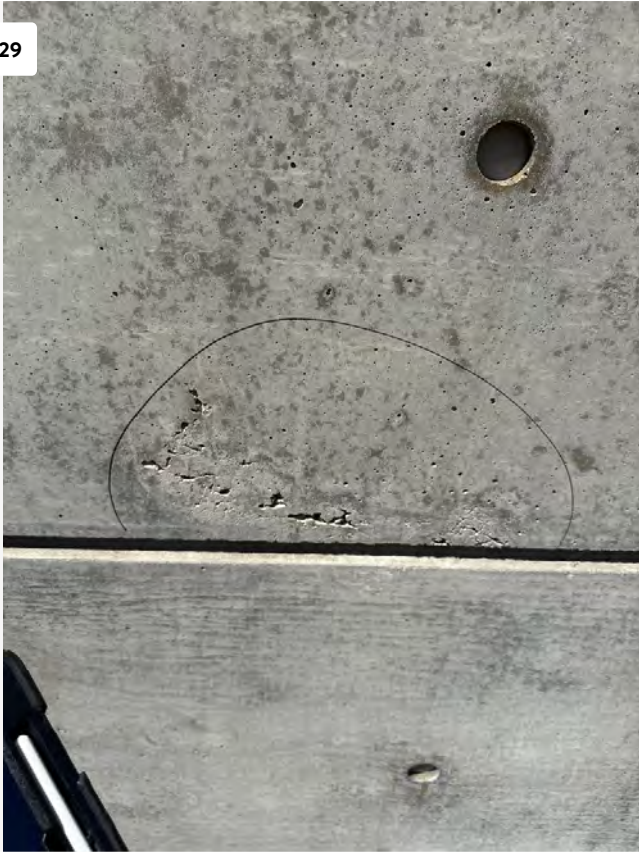
Honey Combed Concrete
