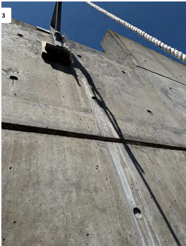
Crack at East Elevation near Parapet
