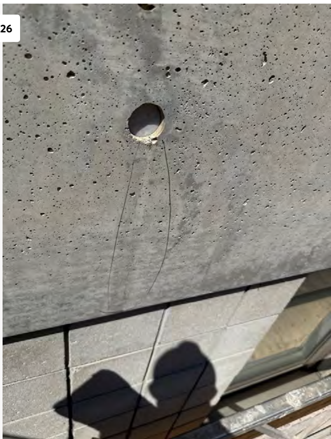
Crack at East Elevation
