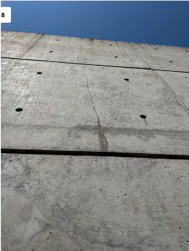
Crack at Bulkhead on East Elevation
