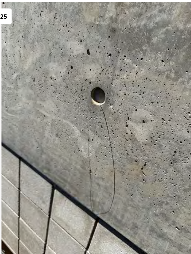
Crack at East Elevation
