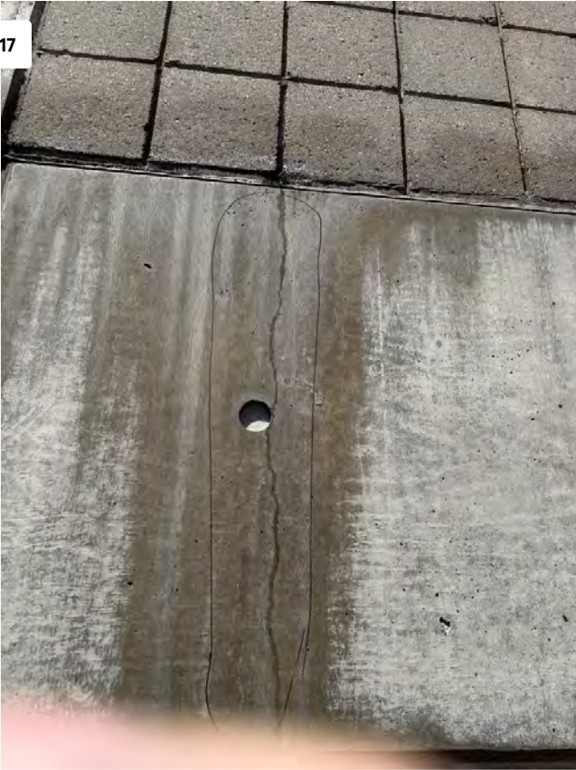
Crack at East Elevation
