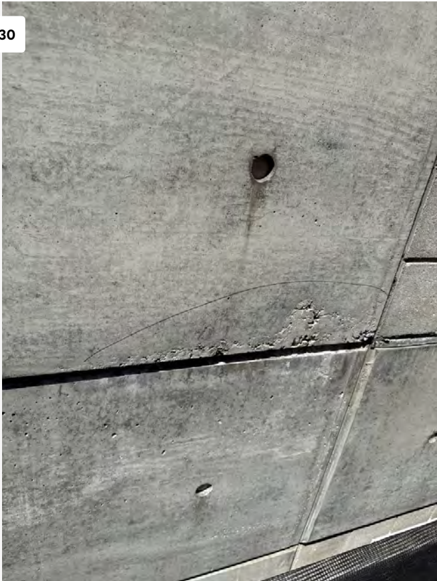
Honey Combed Concrete
