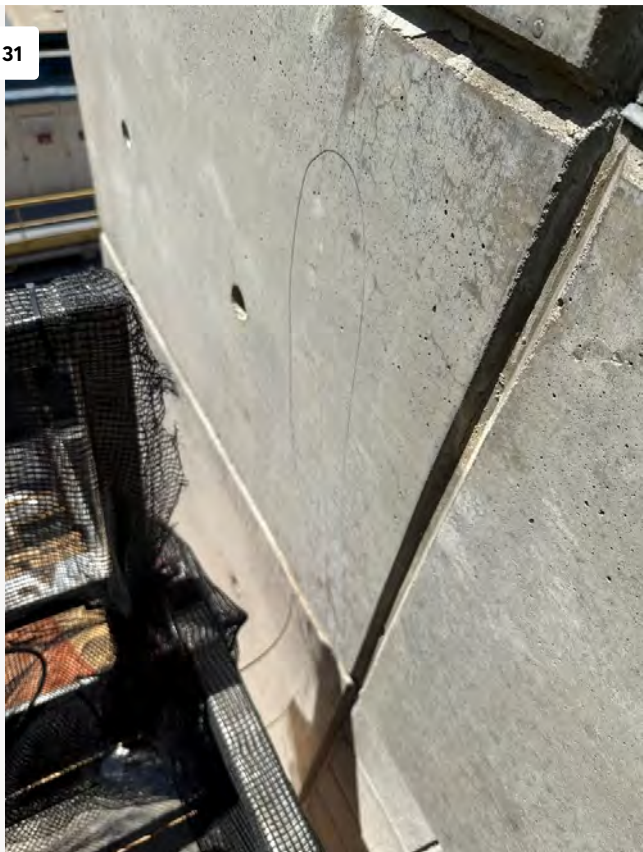
Crack at East Elevation
