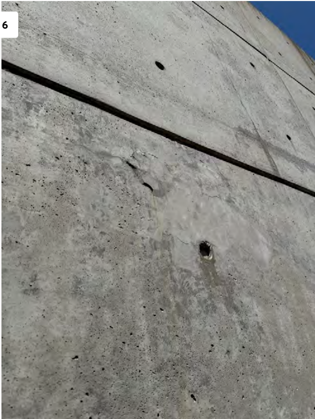
Old Patch that Needs to be Demoed
