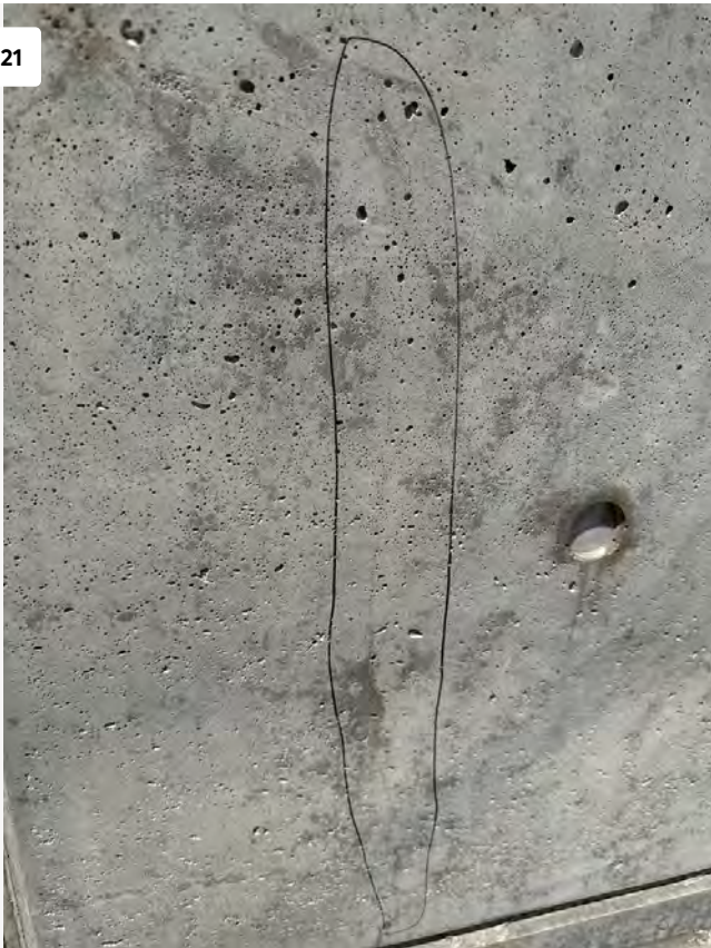
Crack at East Elevation
