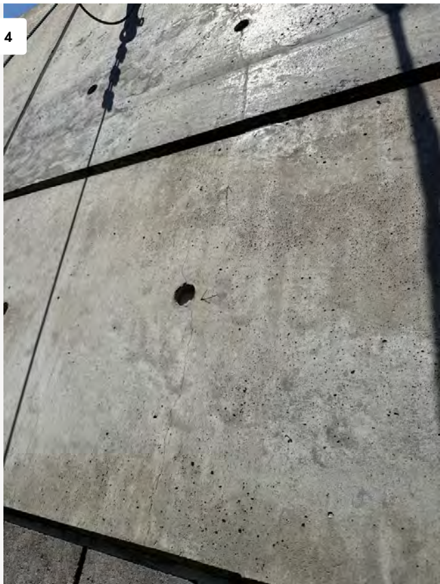
Crack at East Elevation
