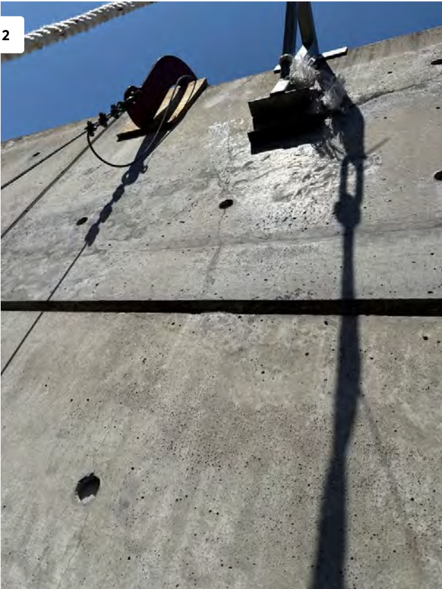
Crack at East Elevation Near Parapet
