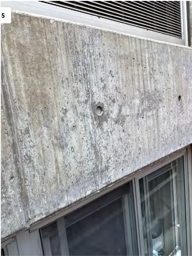
Crack Demoed at North Elevation
