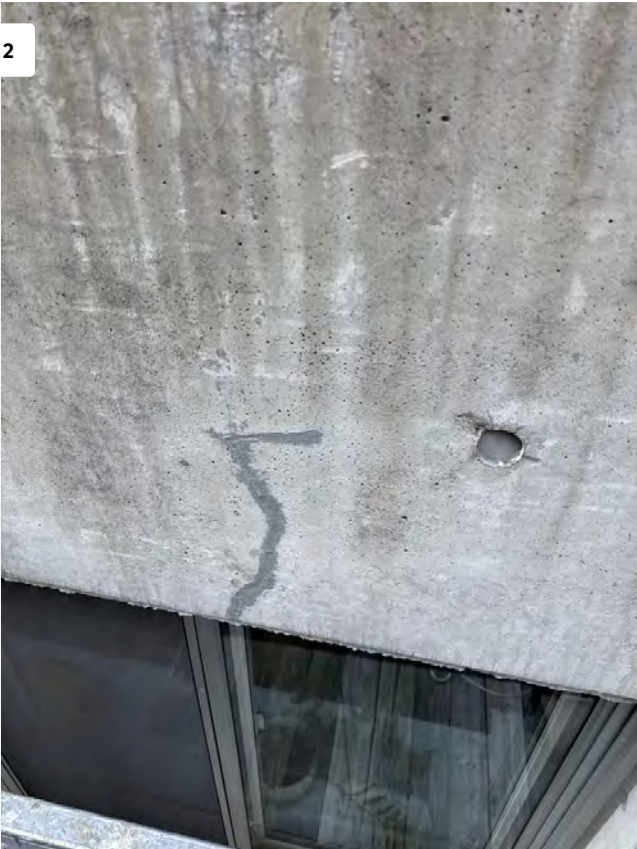
Crack Repair at North Elevation, Crack Still Visible and Will Need to be Addressed
