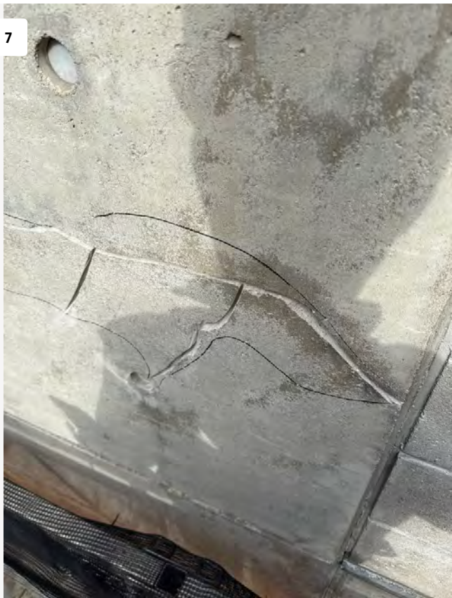
Demolished Crack at East Elevation
