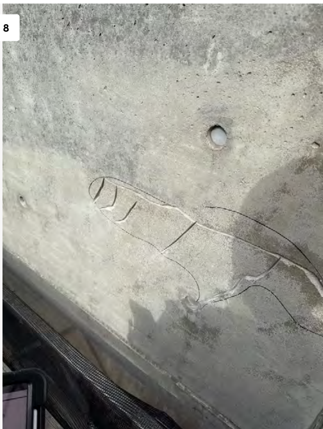
Demolished Crack at East Elevation
