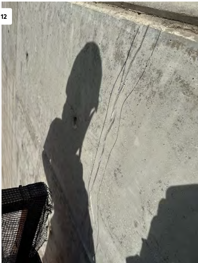
Crack at East Elevation
