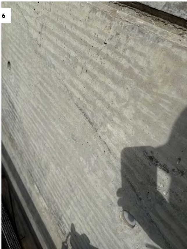
Discoloration at East Elevation
