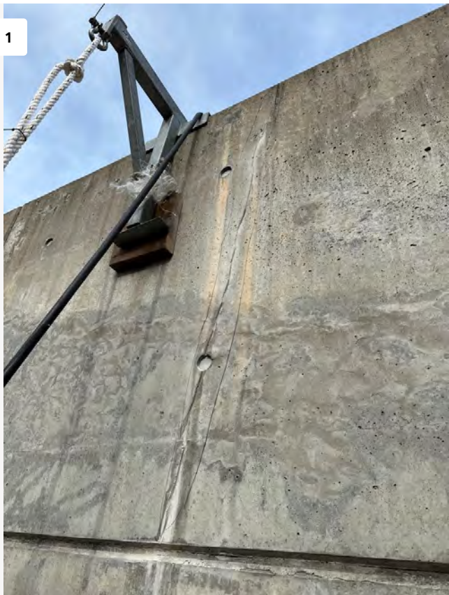
Demolished Crack at East Elevation
