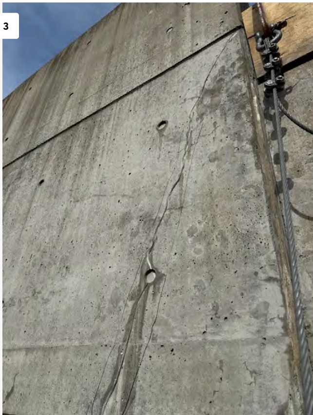
Demolished Crack at East Elevation
