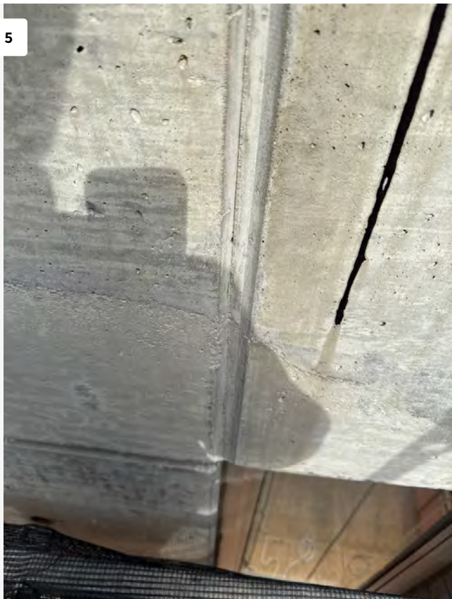
Discoloration at East Elevation
