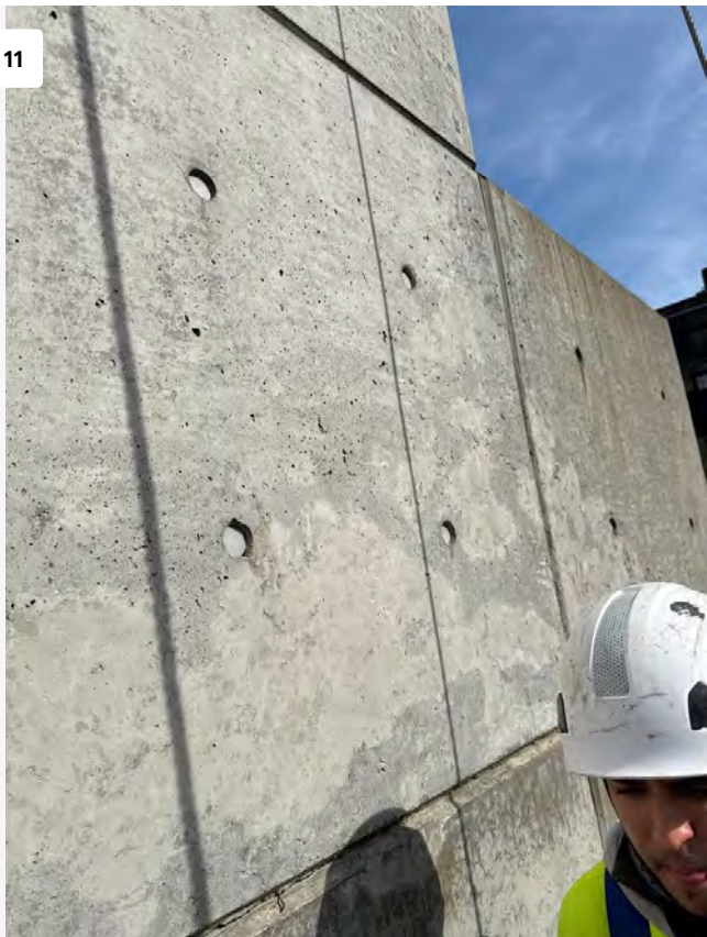
Discoloration at East Elevation
