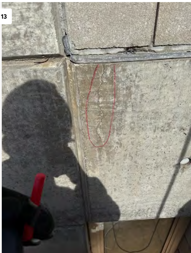
Crack at East Elevation
