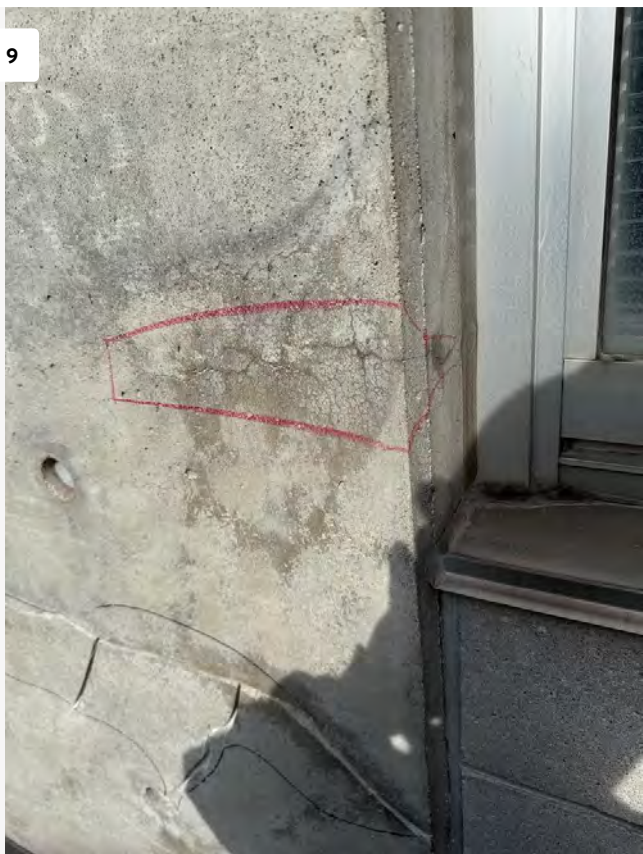
Crack at East Elevation
