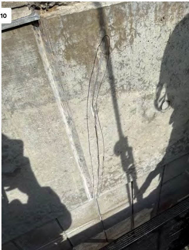
Demolished Crack at East Elevation
