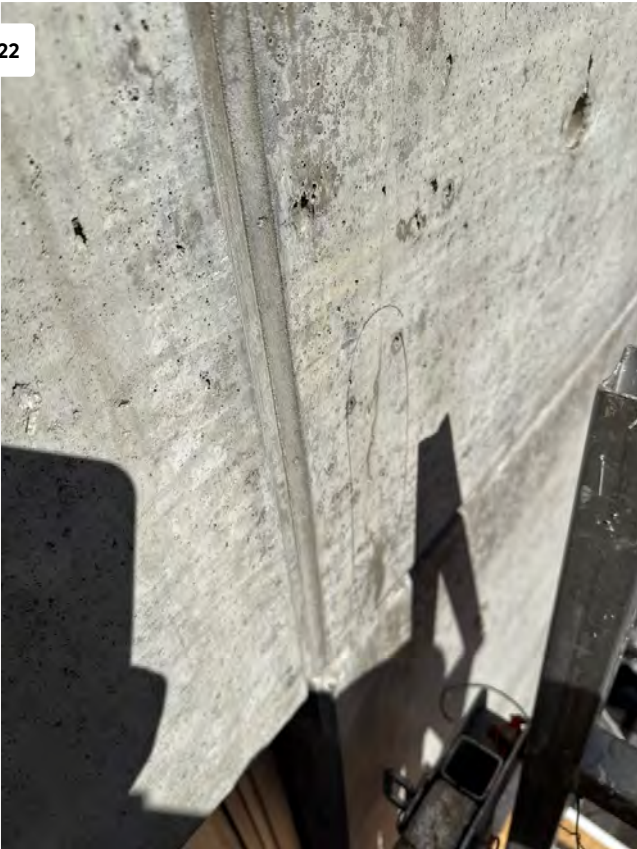
Crack at north elevation
