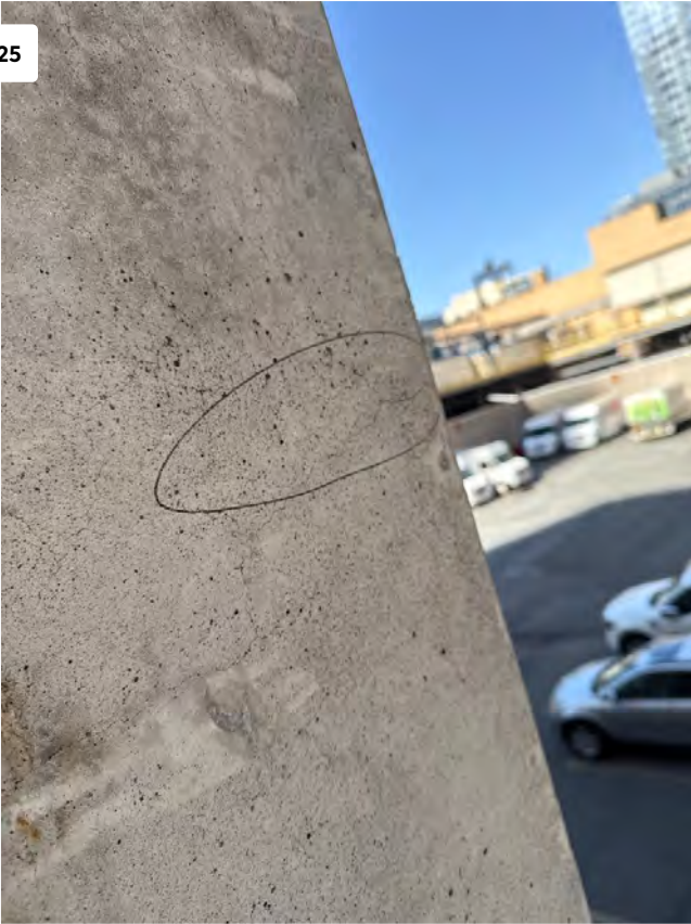
Crack at north elevation
