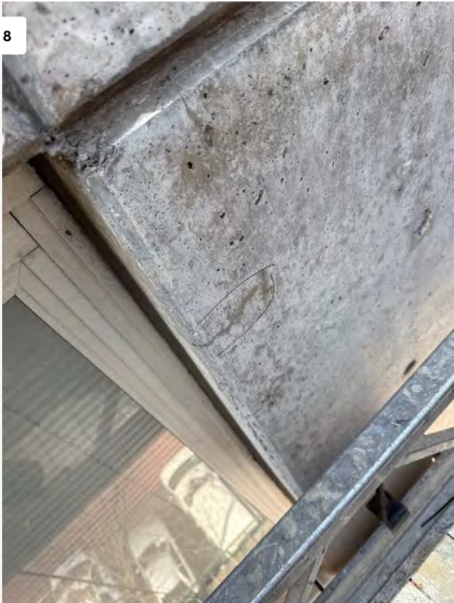
Crack at north elevation
