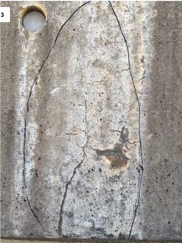
View of Crack at North Elevation.
