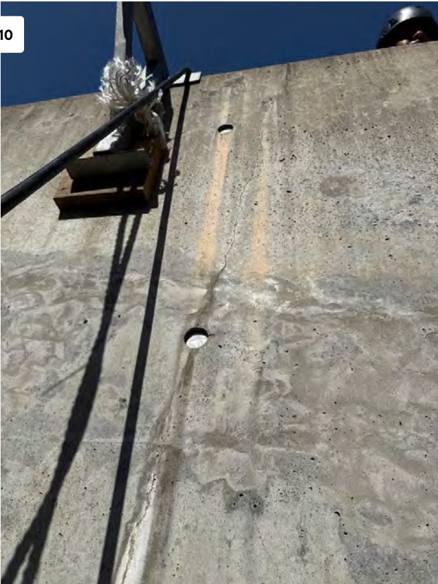
Crack at east elevation
