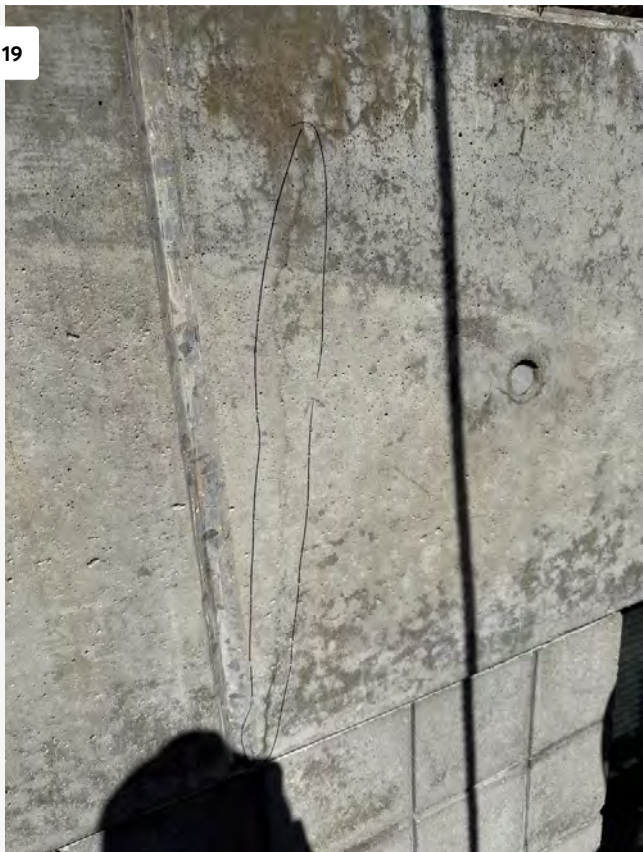
Crack at east elevation
