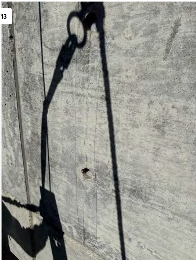
Crack at east elevation
