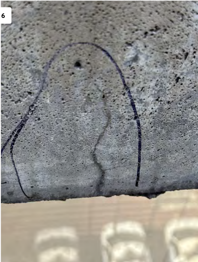
Crack at north elevation
