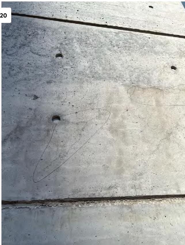
Crack at east elevation
