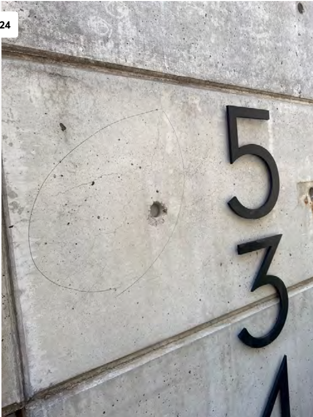
Crack at north elevation
