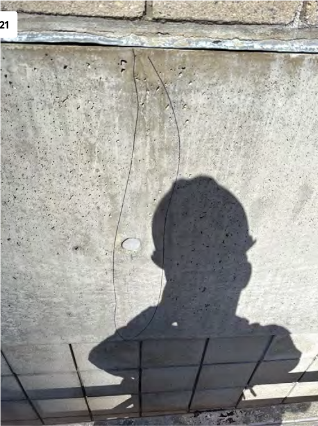
Crack at north elevation
