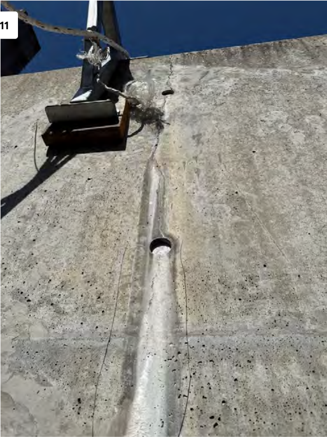
Crack at east elevation
