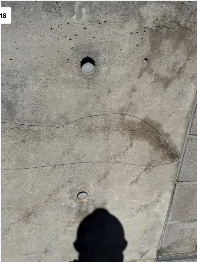
Crack at east elevation
