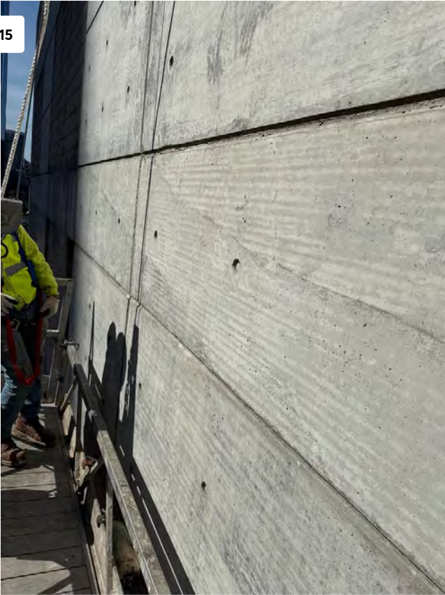
discoloration at east elevation
