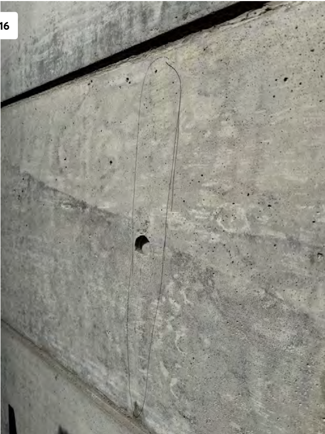
Crack at east elevation
