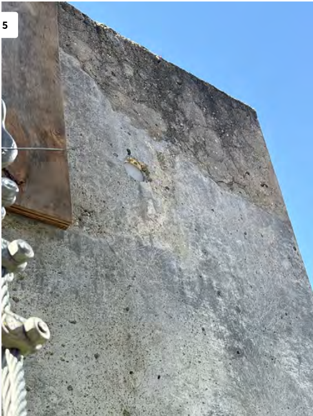
crumbling at north elevation on balcony
