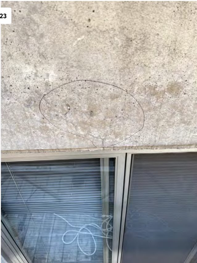
Crack at north elevation
