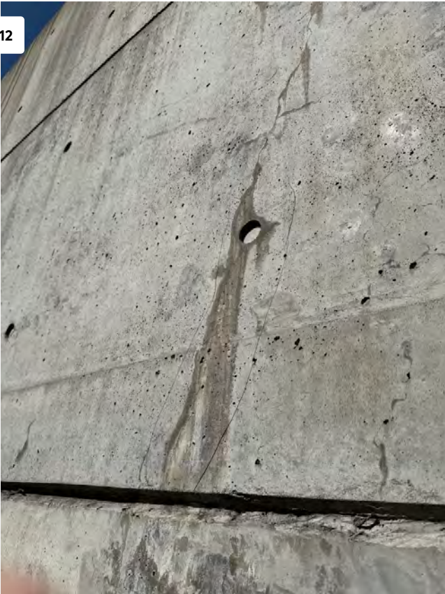
Crack at east elevation
