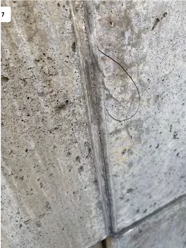
Crack at north elevation
