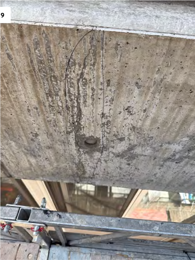
Crack at north elevation
