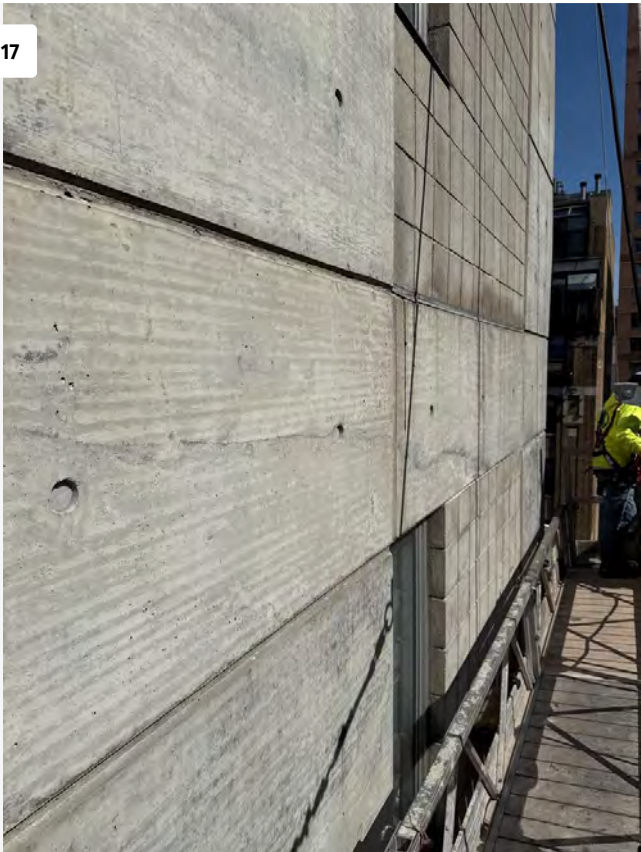
discoloration at east elevation
