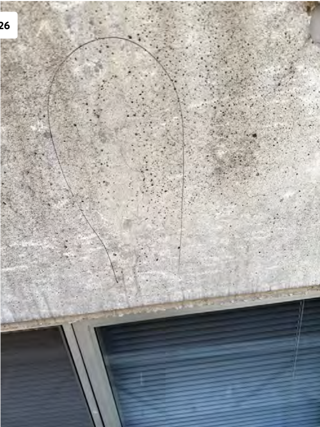
Crack at north elevation
