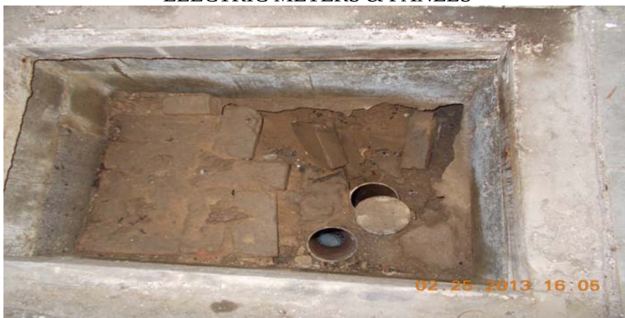
HOUSE TRAP & SEWER CLEANOUT – NEEDS COVERING CLEANOUT
