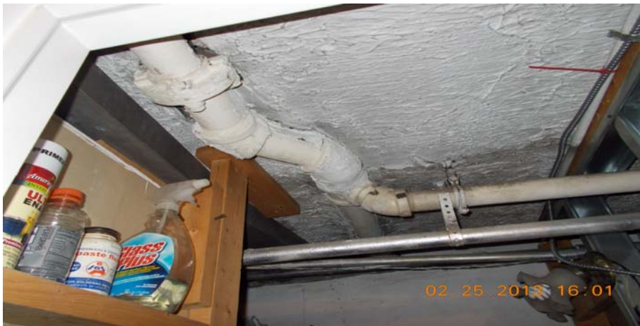
BASEMENT - ASBESTOS ON HEATING PIPES
