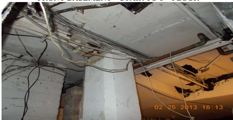
FRONT BASEMENT – COLUMN & LOOSE WIRINGS
