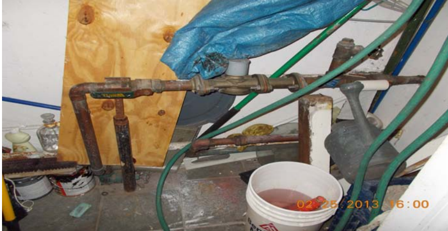
INCOMING WATER MAIN & METER
