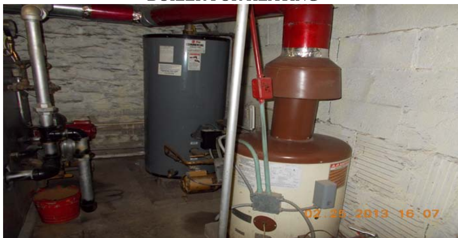
HOT WATER BOILER & STORAGE TANK
