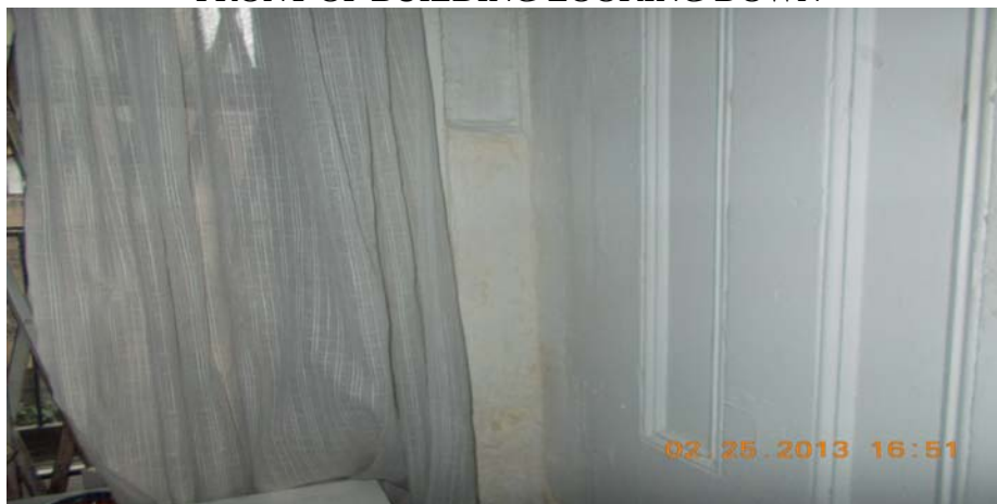
APT. # 2B – REAR KITCHEN WALL – WATER DAMAGES
