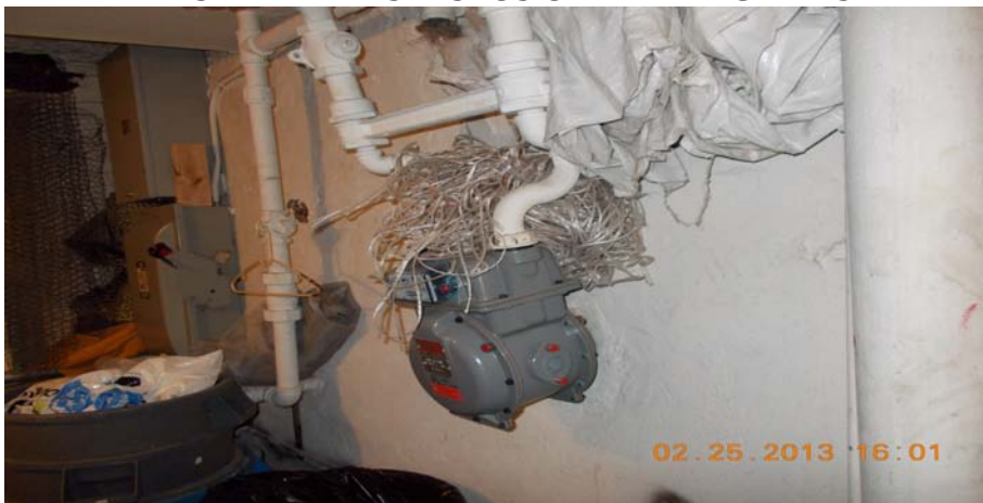
GAS METER FOR BUILDING - HEATING & HOT WATER
