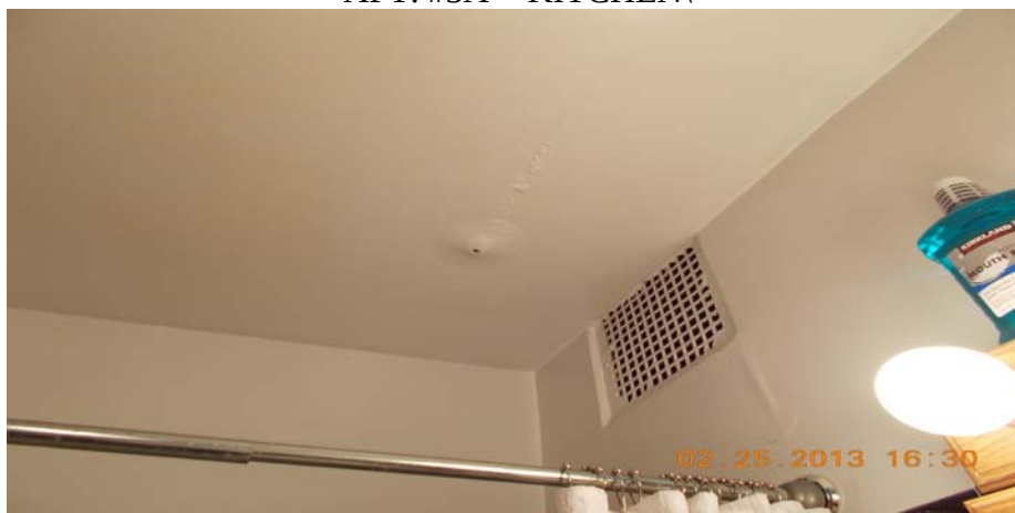
APT. #3A - BATHROOM CEILING - PAST LEAKS
