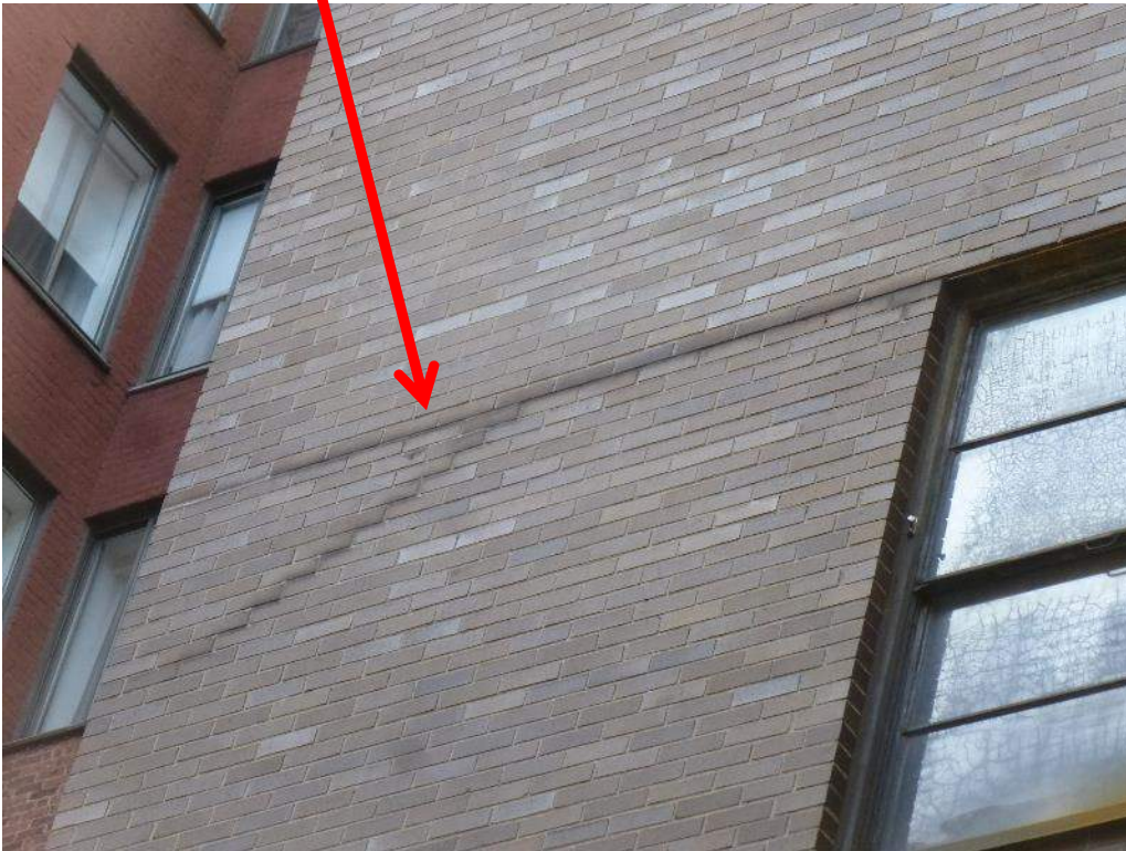
Detail Photo No. 30 – Detail view of cracked brick and loose mortar joints.
