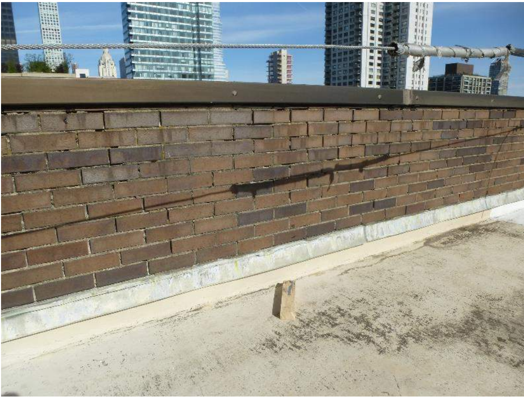
Detail Photo No. 41 – Main Roof parapet – deteriorated mortar joints.
