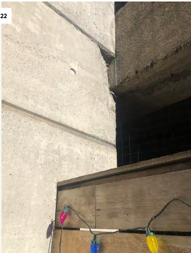
Typical View of Spalling Concrete at South Elevation noted in Initial & Subsequent 9th Cycle FISP Report Filings.
