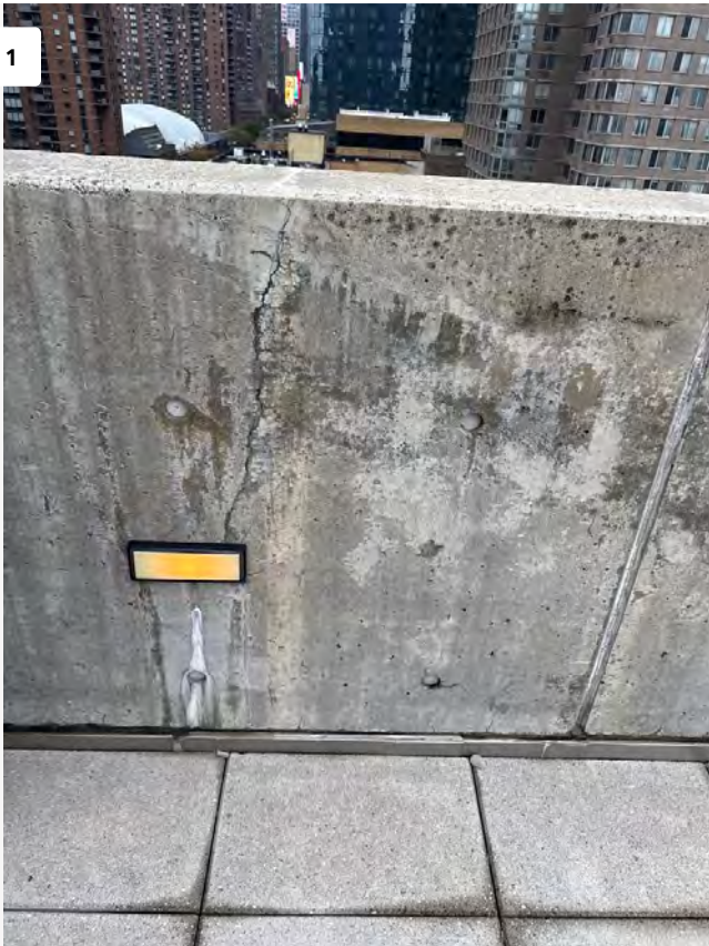
Typical View of Cracked Concrete at Parapet noted in Initial & Subsequent 9th Cycle FISP Report Filings.
