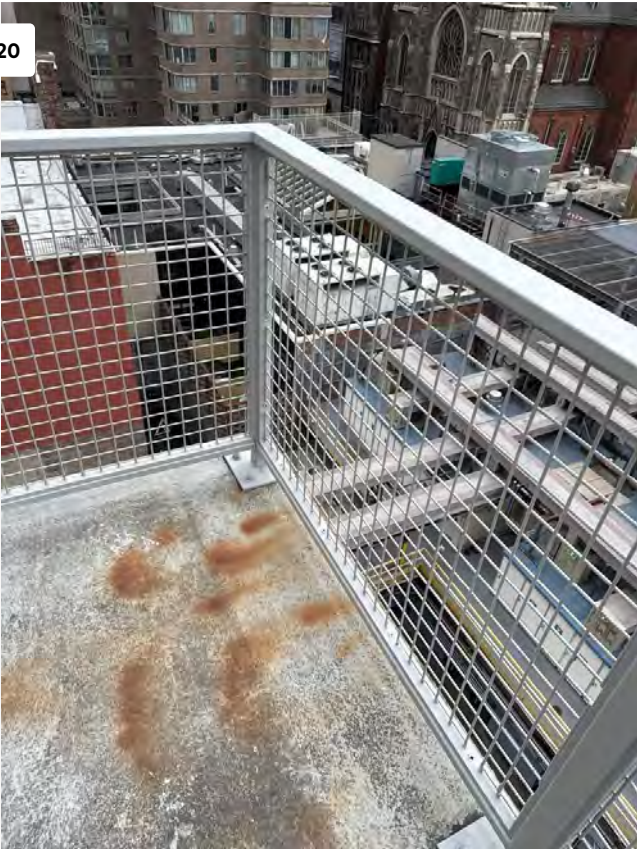
Typical View of Scraped, Primed, and Painted Surface Rust at Balcony Railing along South Elevation.
