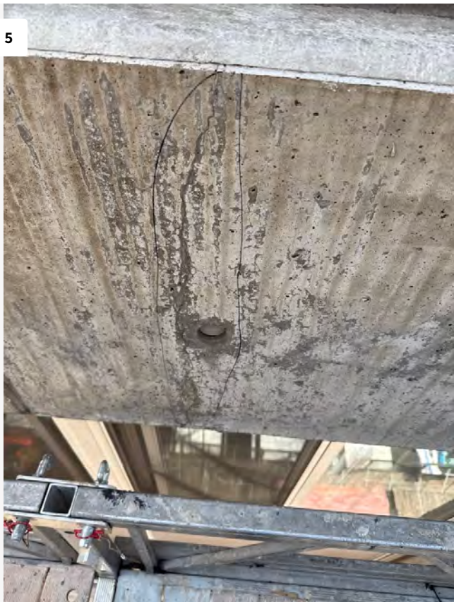
Typical View of Cracked Concrete at North Elevation noted in Initial & Subsequent 9th Cycle FISP Report Filings.
