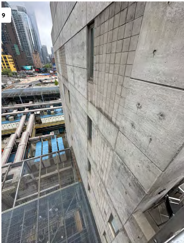
Typical View of Cracked Concrete at East Elevation noted in Initial & Subsequent 9th Cycle FISP Report Filings.
